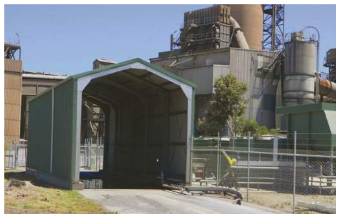
The new Elder Road truck wash system installed at the Birkenhead plant.
