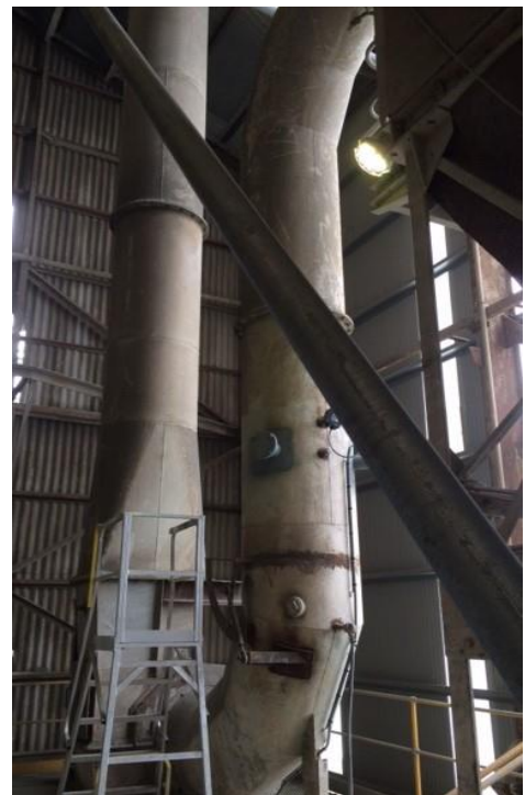
Figure 2: Cement Mill 2 Exhaust Duct
