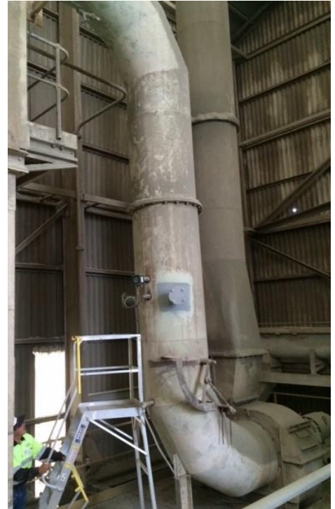
Figure 1: Cement Mill 1 Exhaust Duct
