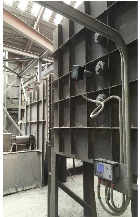
Figure 3: Cement Mill 3 Exhaust Duct
