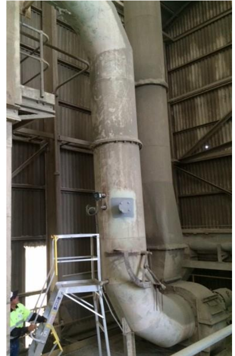
Figure 1: Cement Mill 1 Exhaust Duct
