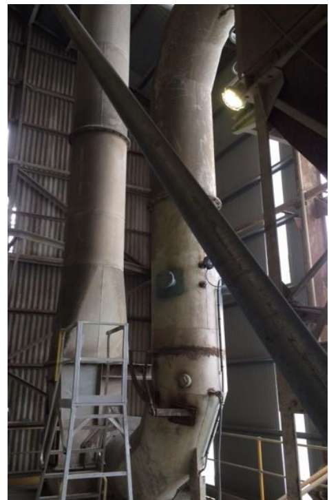
Figure 2: Cement Mill 2 Exhaust Duct
