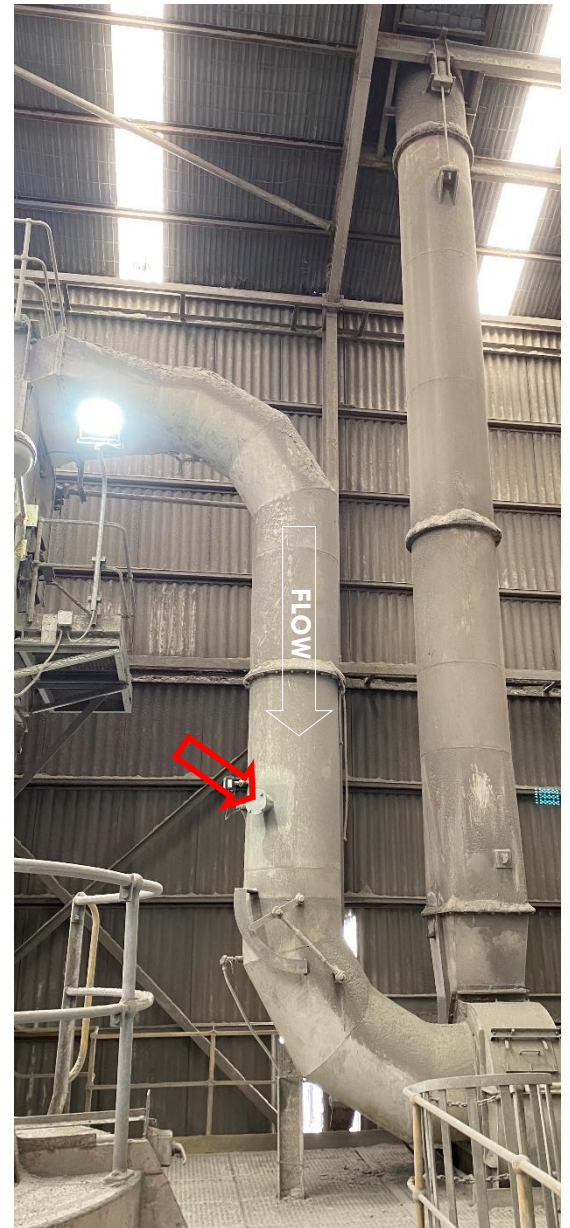
Figure 2: Cement Mill 1 Exhaust Stack sampling location
